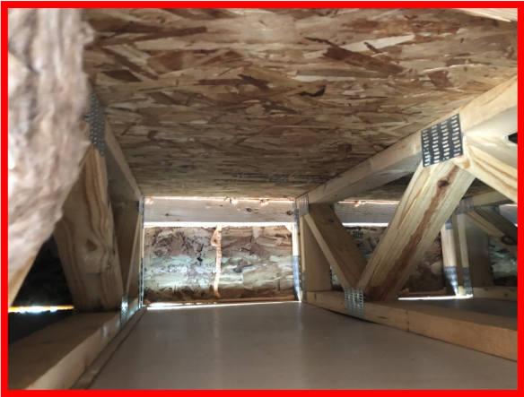
NOT sealed, no insulation
