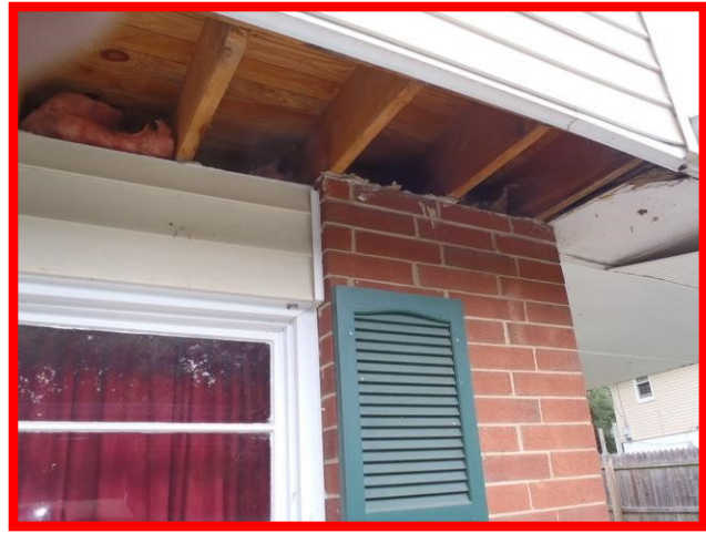
Open bays, not enough insulation
